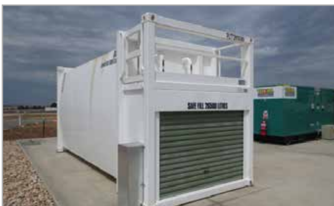
Liquitainer being used for Generators
